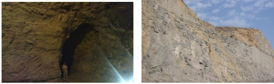
Figure2. Geological survey at preconstruction stage on outcrops and slopes (right) at construction stage in tunnel route (left) [8]
